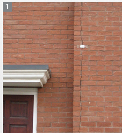
1 Cracking resulting from thermal expansion and contraction
